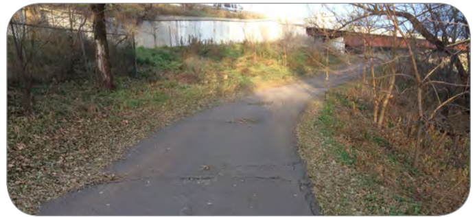
Subsegment D4 is scheduled for reconstruction in 2022. The I-694 underpass can be seen in the distance, which also requires upgrades (as noted in Subsegment D3). Source: Three Rivers Park District
