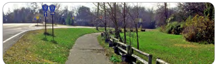
The existing Segment A2 pavement requires maintenance including short-term patching and sealing with mid to long term plans to replace.
